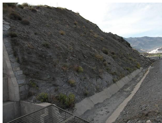
Figure 3. Embankment in the kilometric point 339 belonging to the A92 dual carriageway, Spain
