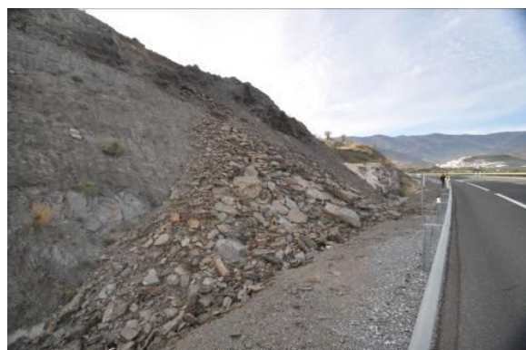
Figure 4. Landslide detail with the contention wall in the second plane of the image
