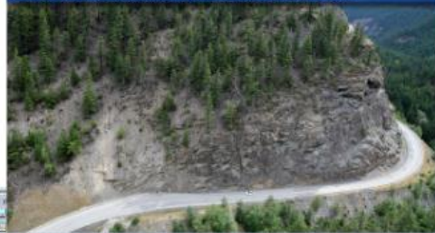
Photo of a bluff requiring rock slope remediation. Part of a government remediation project, this photo will be one of many used to calculate the mesh area and other
